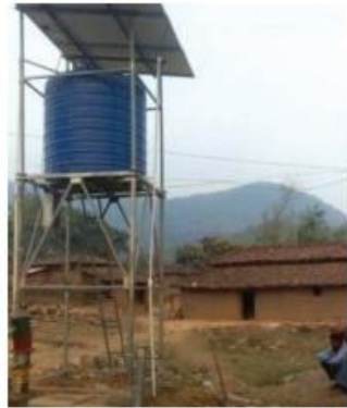
Solar light and pump
